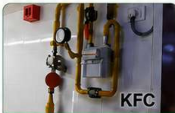
Flow Meter Installation at KFC Outlet
