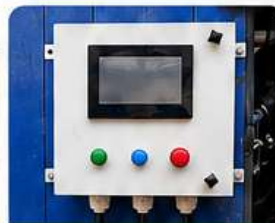
DUAL FUEL CONTROL PANEL
