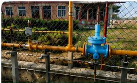
PRESSURE REGULATING STATION
