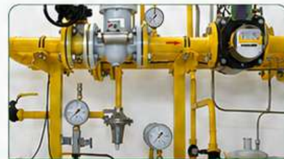
Flow Meter Installed in LPG Pipeline System
